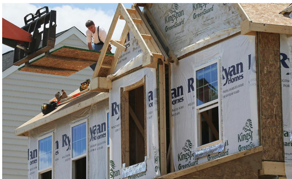
In this Thursday, June 1, 2017, photo, builders work on the roof of a home under construction at a housing plan in Jackson Township, Butler County, Pa. (AP Photo/Keith Srakocic)
